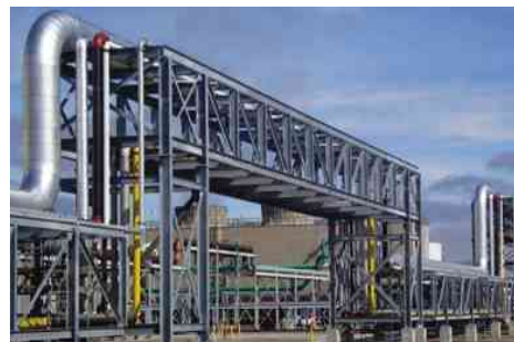
Pipe Support Structures
