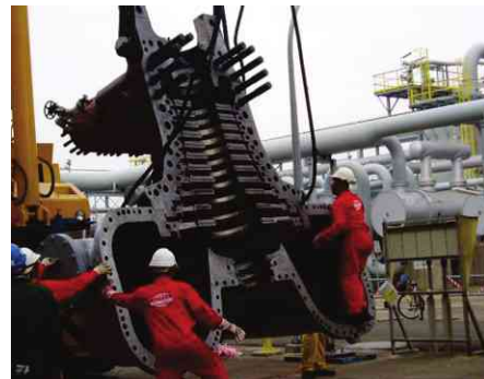
Part of a Steam Turbine
